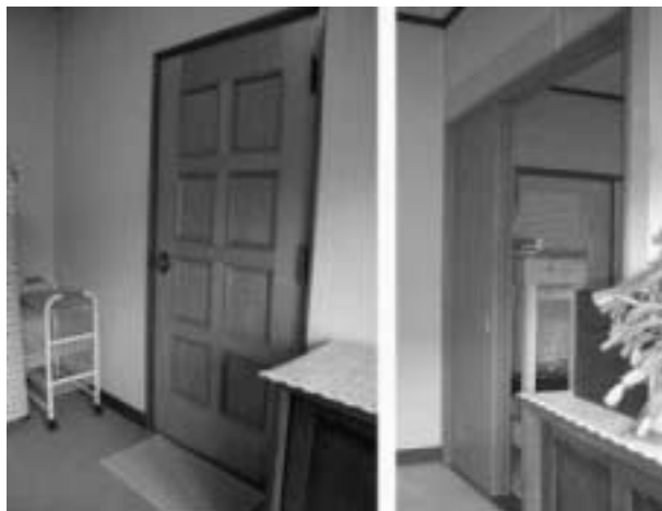
図8 居室への出入り口(左:改造前,右:改造後) Fig.8 Remodel a door (Left: before, Right: after)
